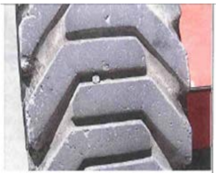
Bolt in tyre – this is not a fault – bolt is used to plug their air hole after filling
